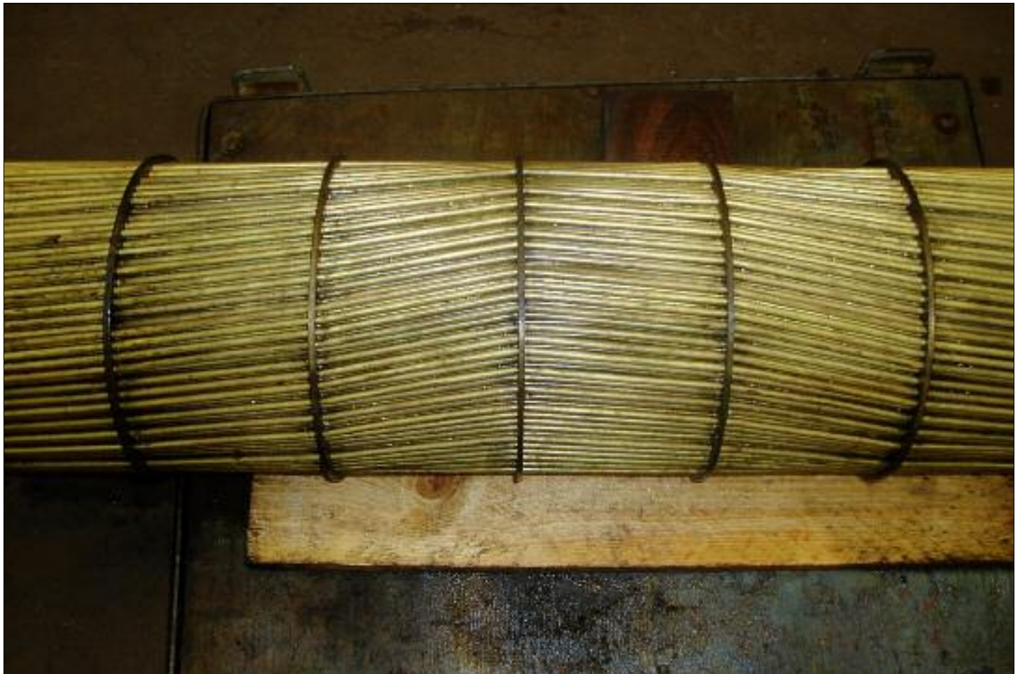
33 002's stripped down heat exchanger showing the frost damage distortion to the internal tubes June 2007
